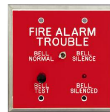
Fire Alarm Trouble
