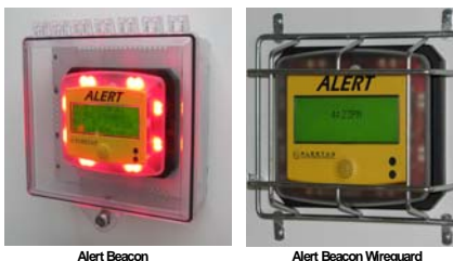
Figure 1 Alert Beacon Installed in an Outdoor Enclosure and an Alert Beacon Wireguard
