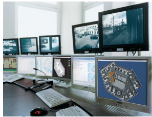
Control center, security company
