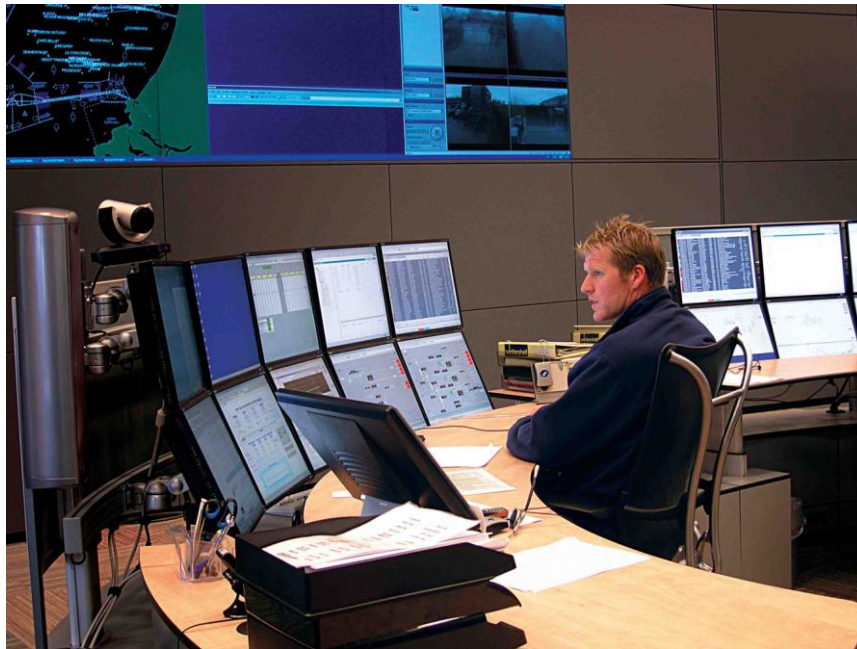
Figure 3. Modern HMIs have allowed operators to become intimately involved in plant operations.
