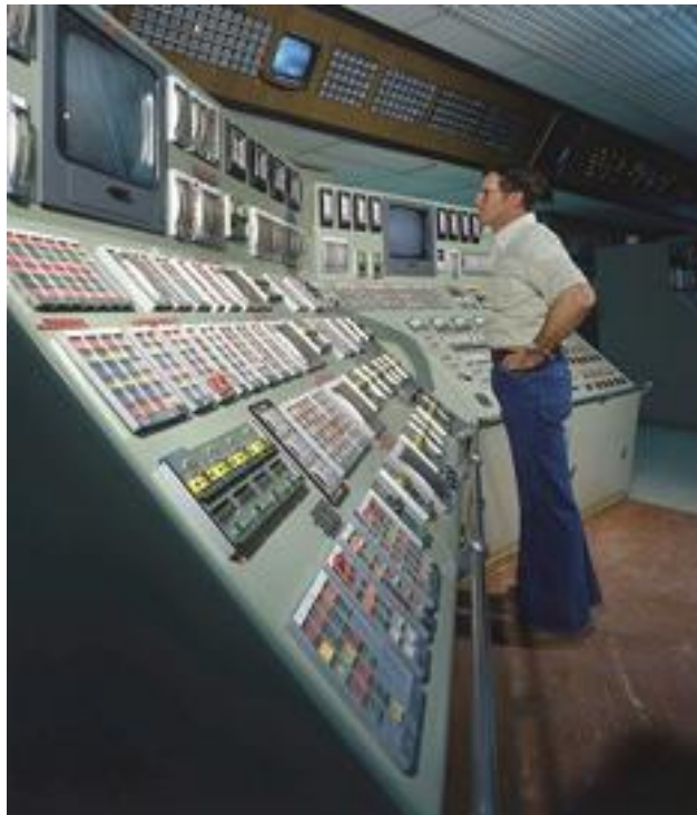
Figure 2. Early control room panel boards featured mechanical pushbuttons and an array of warning lights.
