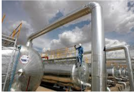
Gas Transport & Storage at Hazira
