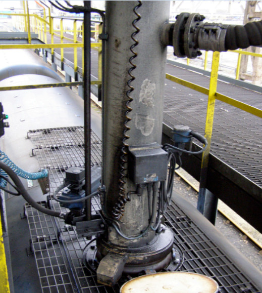
View of Conoco Phillips-Humber Refinery, UK - rail loading operation, powered by Terminal Manager
