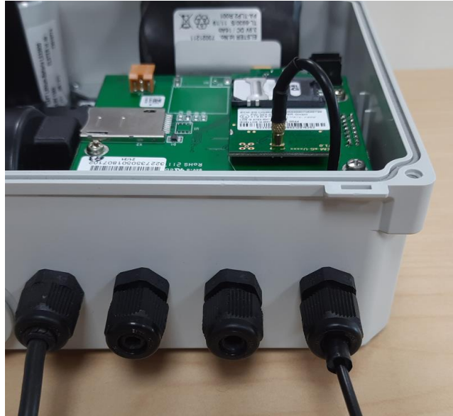
Fig. 34: External antenna connected to modem assembly
