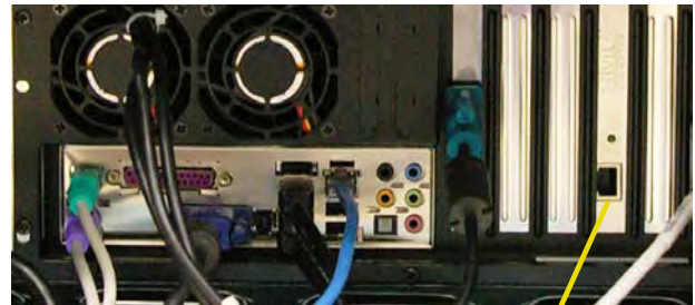
External Ethernet Connection
